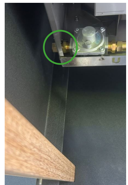
3. Connection point beneath the BBQ. Remove the installed adapter, circled.
